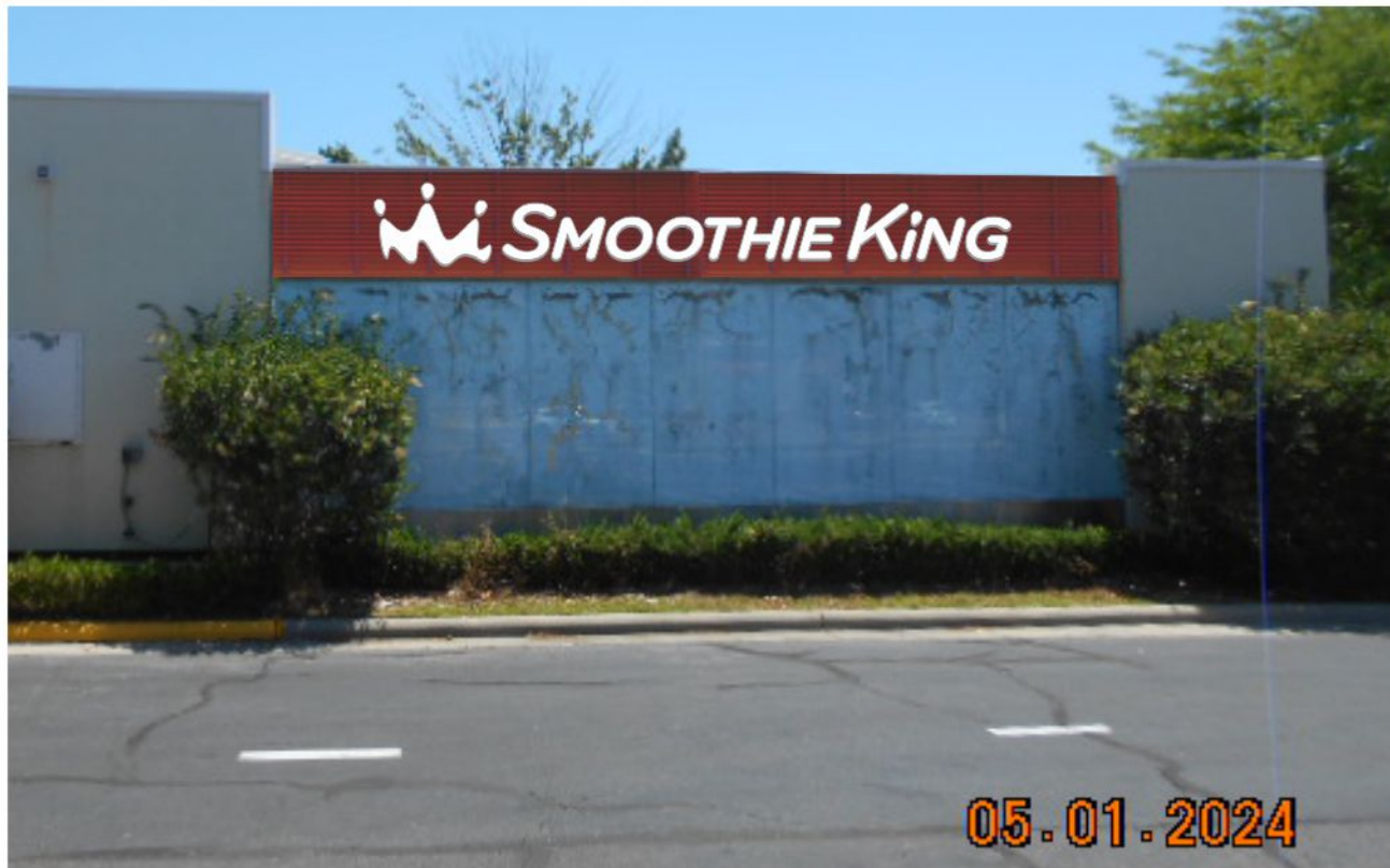
Tube grid wall is to be painted SW 7593 Rustic Red by others.
