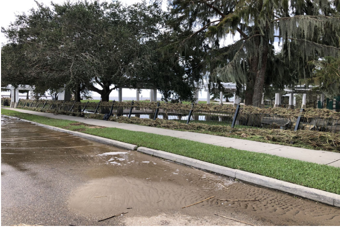
Photo Depicts Aluminum Ornamental fence damaged from storm debris.
