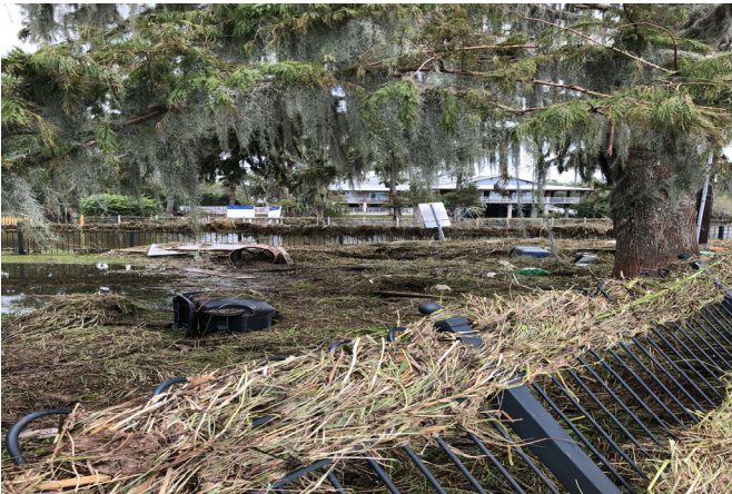
Photo Depicts another view of Aluminum Ornamental fence damaged from storm debris.
