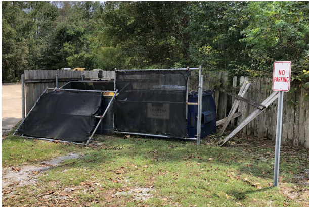
Photo Depicts wooden Dumpster enclosure with Galvanized posts. In addition, Galvanized fabricated gate.
