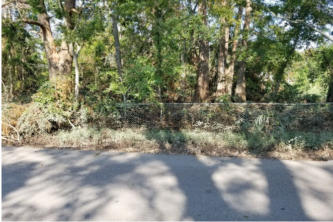
Photo Depicts chain-link fence damaged from storm debris.
