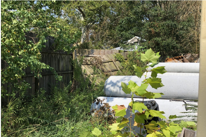
Photo Depicts wooden fence leaning and damaged.
