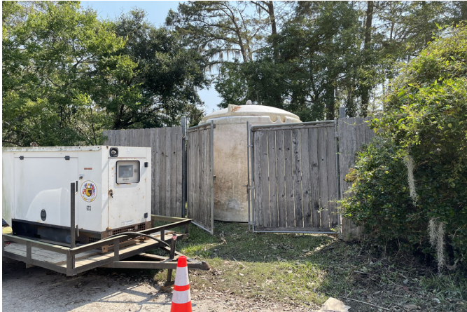
Photo Depicts gate sagging due to leaning posts.
