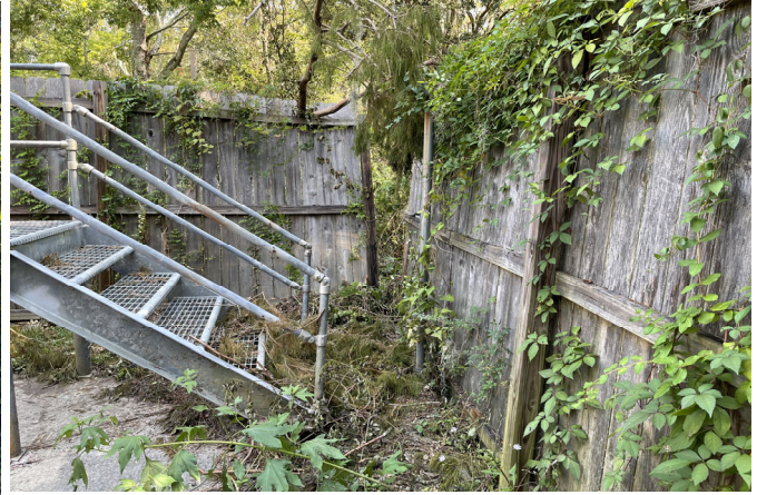
Photo Depicts wooden fence leaning and damaged.
