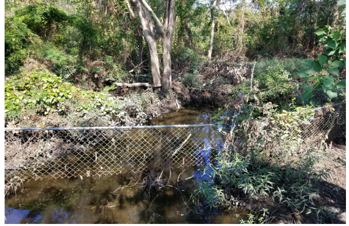
Photo Depicts sunken fence posts.
