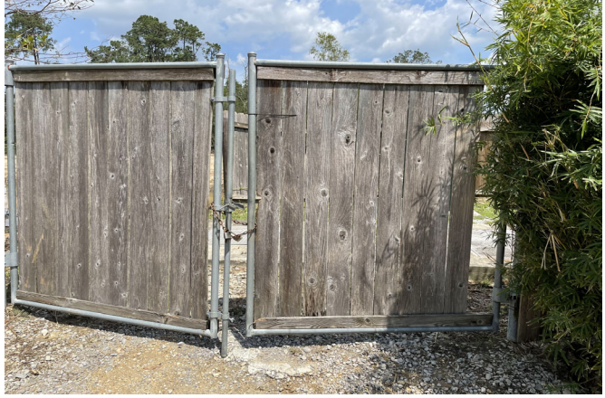
Photo Depicts gate missing fence boards.
