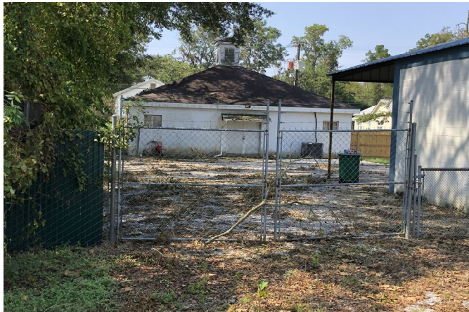
Photo depicts sagging/damaged chainlink fence.
