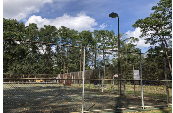
Phot depicts Tennis court fence fabric damage.
