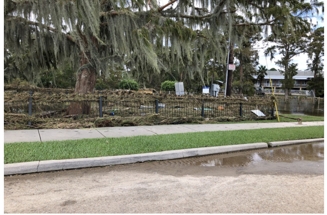
Photo Depicts another view of Aluminum Ornamental fence damaged from storm debris.
