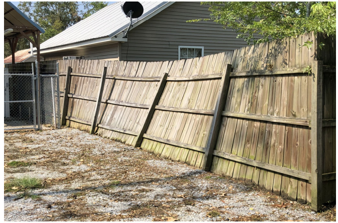
Photo Depicts wooden gate leaning and damaged
