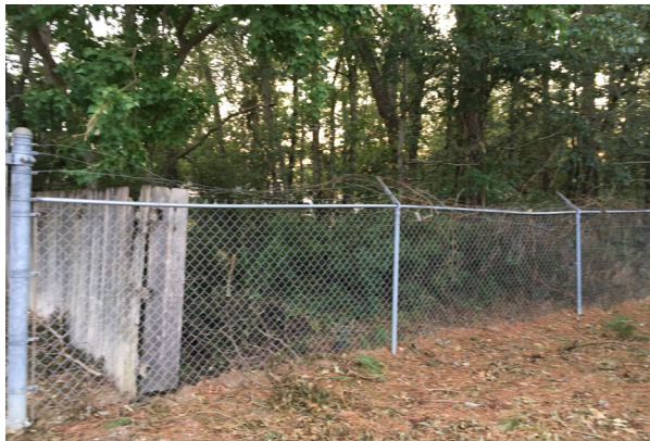
Photo Depicts barbed wire damaged.
