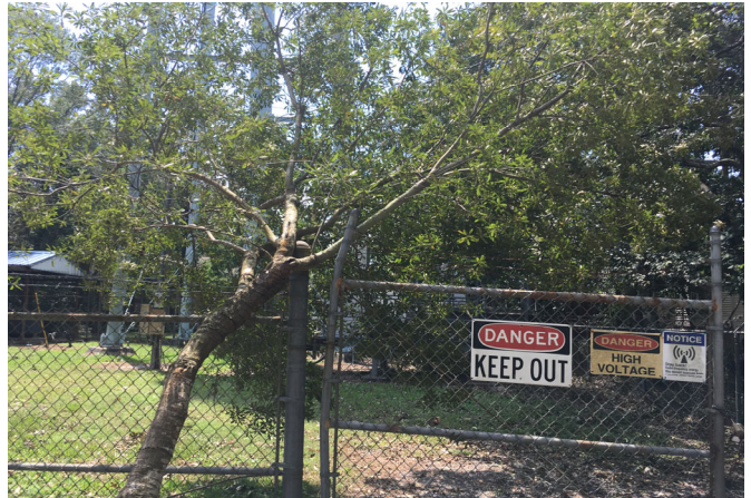
Photo Depicts fence and gate damaged from debris.
