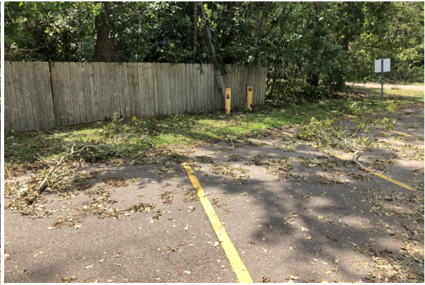
Photo Depicts damaged and leaning wooden fence.
