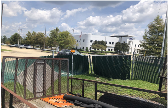
Photo Depicts chain-link fence damaged from storm debris.
