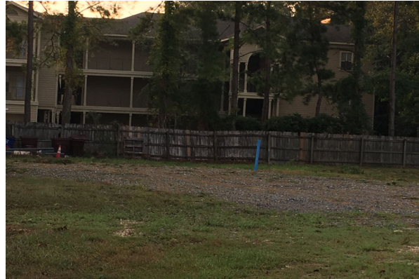
Photo Depicts Wooden Fence damaged and leaning.
